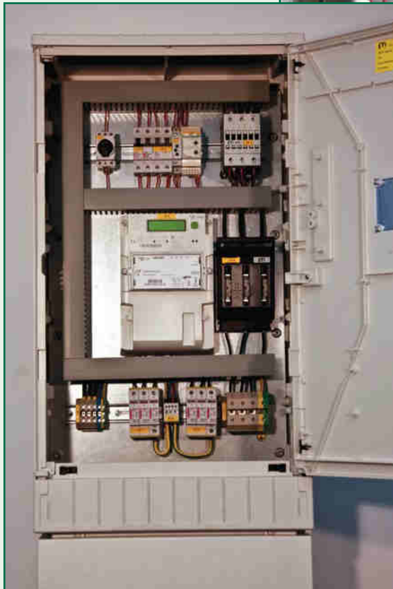
Meter distribution cabinet
