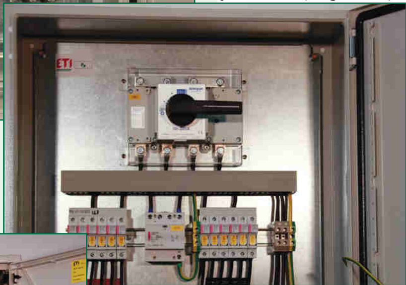
DC junction box (CH gPV fuses)
