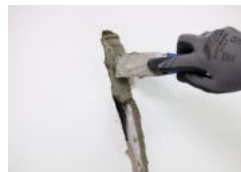
Close the damaged area discreetly.
